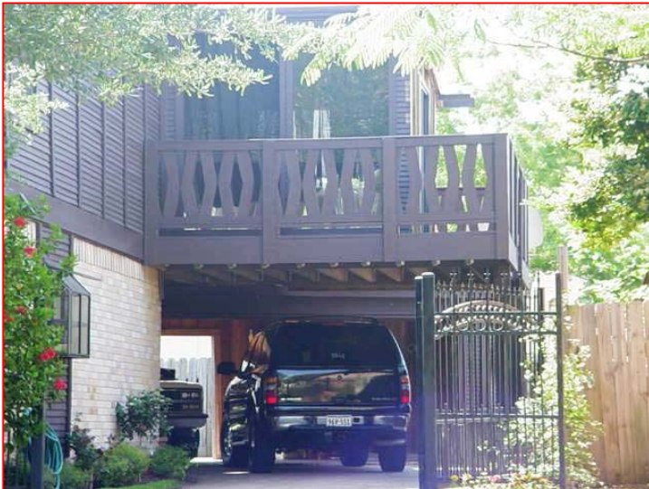
Unapproved addition with encroachment
