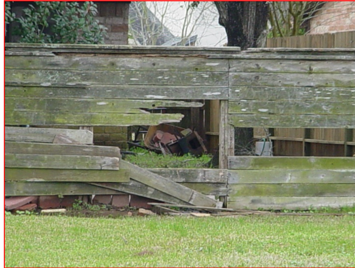
Fence replacement needed & trash in backyard
