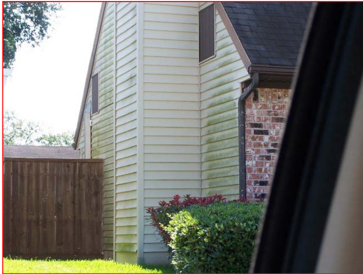
Excessive mildew on siding
