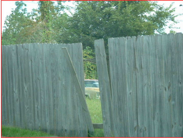
Fence, junk car in back yard, overgrown back yard
